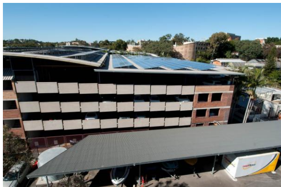
FIGURE 11: The M90 (bottom right) installed next to a 340kW-peak solar array at the University of Queensland
